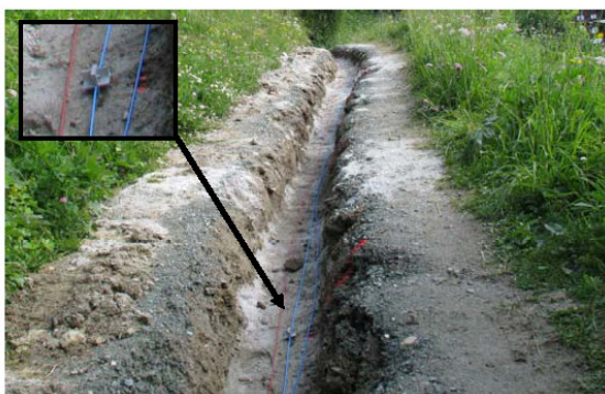
Figure 8. The trench cut in the hiking path with the sensor system already embedded.
