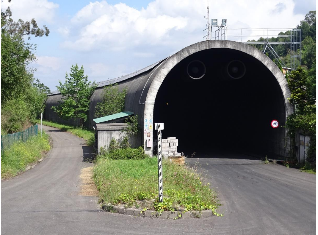
Figure 40: South portal San Pedro des Anes with jet fans
