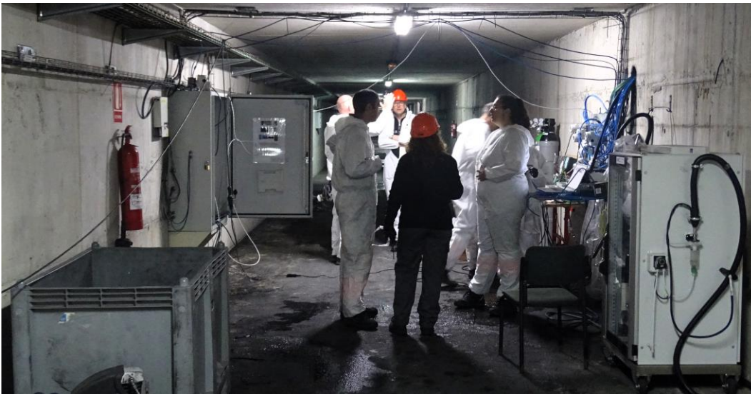
Figure 52: Installation of the heat release rate measurement in the service tunnel at PK522
