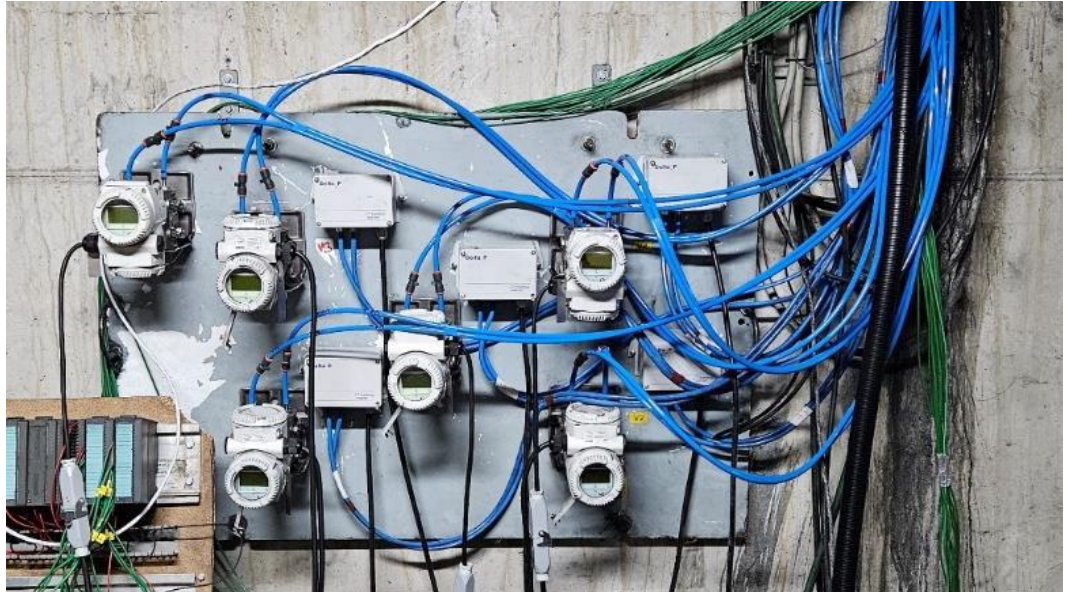
Figure 49: Differential pressure monitors for airflow measurement at pk.522 (located in the service gallery)
