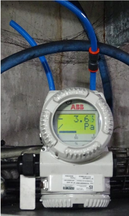
Figure 50: Differential pressure monitor (located in the service gallery)
