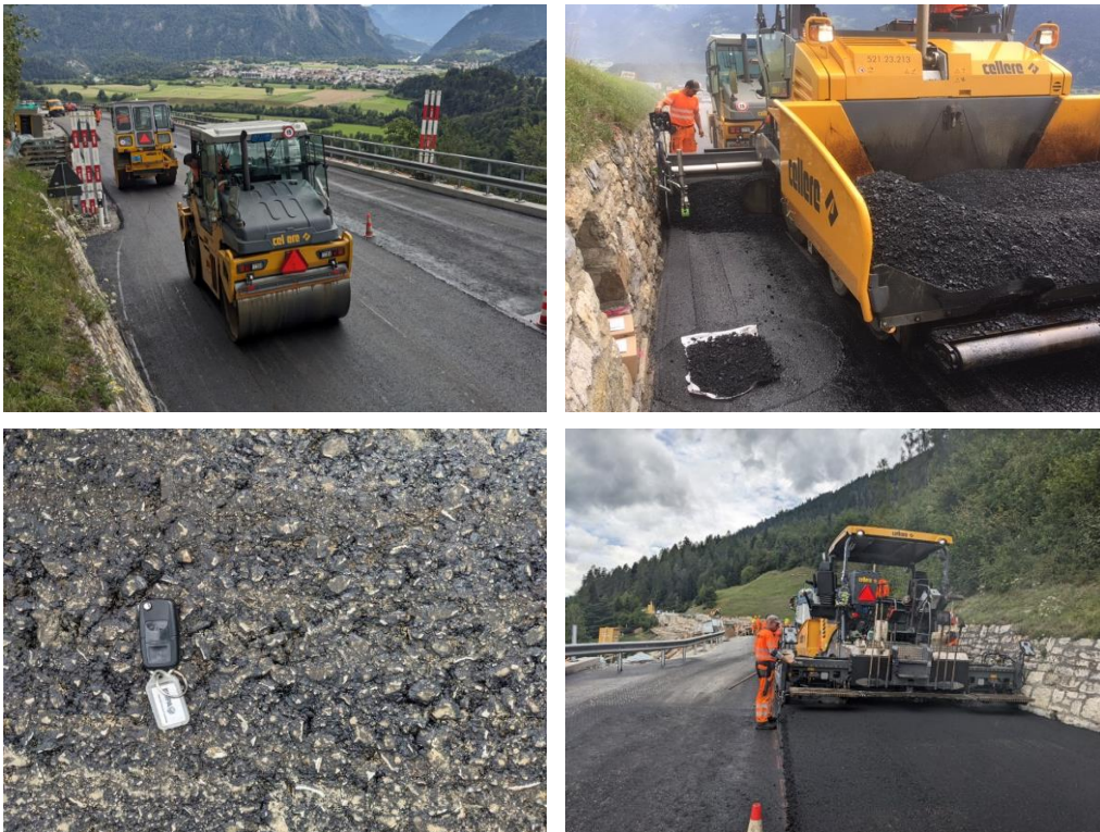
Figure 79: Construction of the AC T 22 S pavement in Tamins – Val Maliens test section
