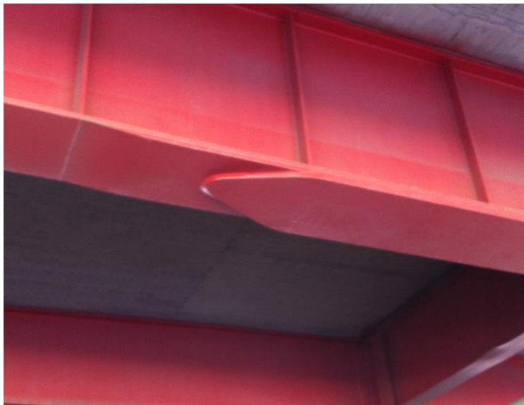
Fig. 53 The critical detail: welded cover plate (located on the 1961 bridge).
