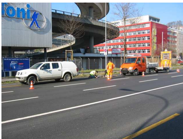
Fig. 4.7: Typical installation of a sampling site (here: Duttweilerstrasse) with trucks and signalization.
