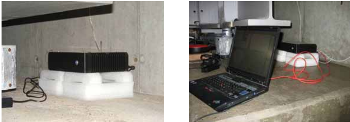
Figure 76: (left) Base-station located under the bridge deck. (right) Laptop running the operator console is directly connected to the base-station in order to access the WSN on-site.
