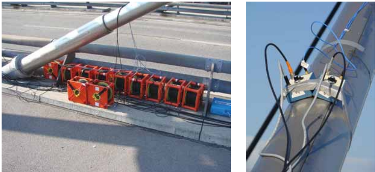
Figure 2: Cabling in the traditional wired SHM installation (2).
