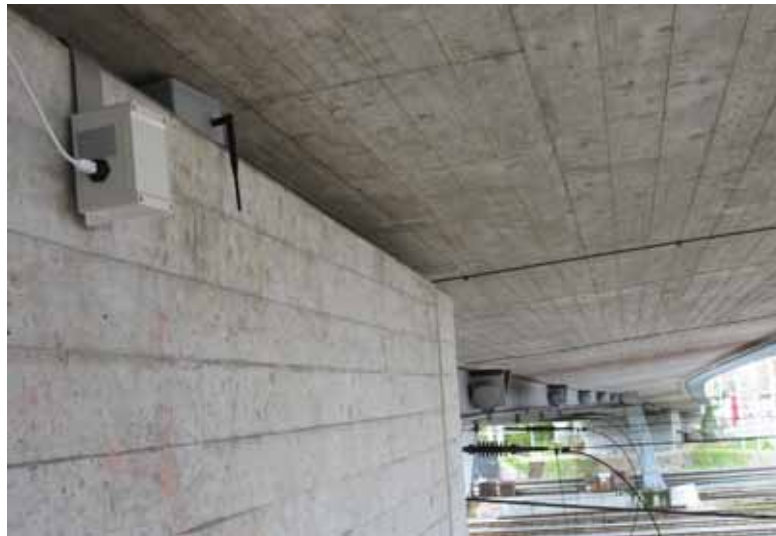
Figure 75: Root node located under the bridge deck.
