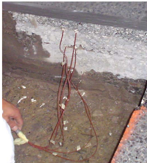
Figure 8. 1: Photograph from installation of temperature sensors showing their location in the pavement
