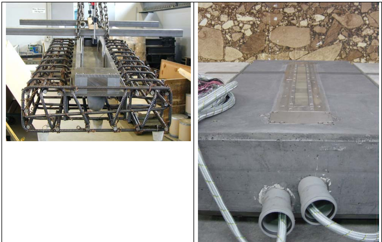
Figure 6. 12: Reinforcement and steel frame of the concrete element (left) and the modulas installed in the concrete element (right)
