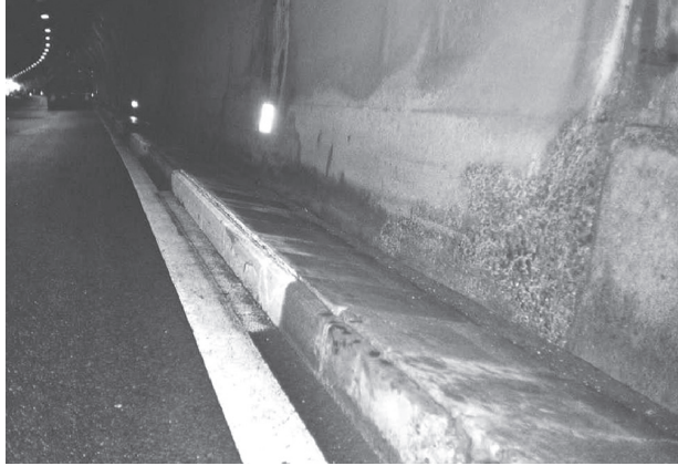
Fig. 2.11. Invert heave and side wall foundation deformation (courtesy of État de Vaud).
